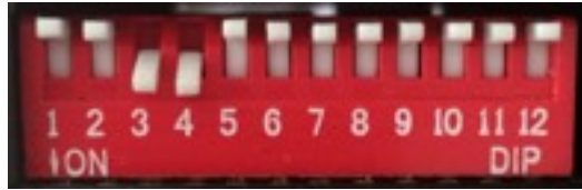
COMMUNICATION SWITCHES PLACE 3, 4 DOWN
